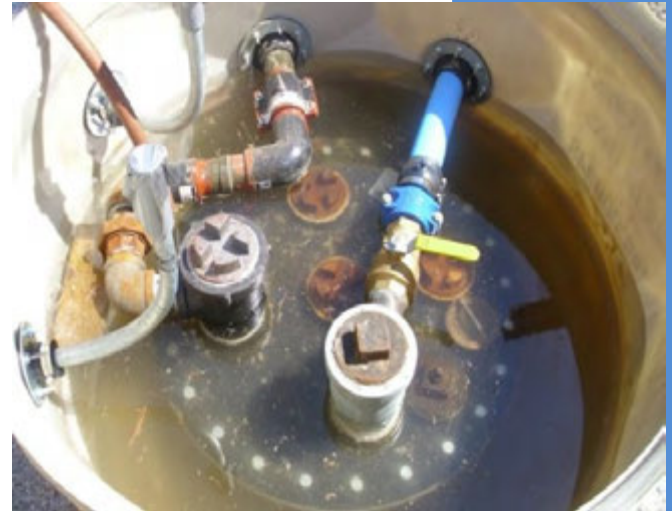
Figure 3.12: Product from double-walled piping collecting in a tank top sump
