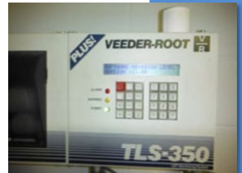
Figure 3.25: Typical monitoring system console
