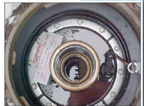
Figure 7.3: View of a flapper valve from a spill bucket
