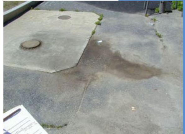
Figure 14.2: Stain from a spill that was not immediately cleaned up
