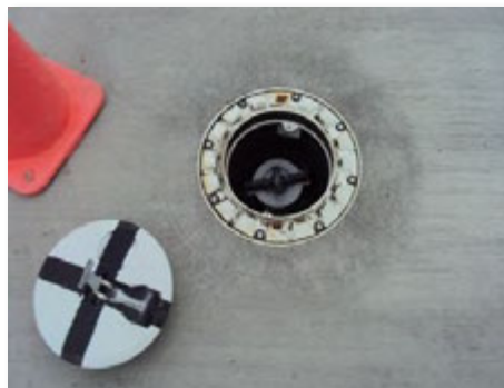
Figure 13.2: Fill port inside spill bucket
