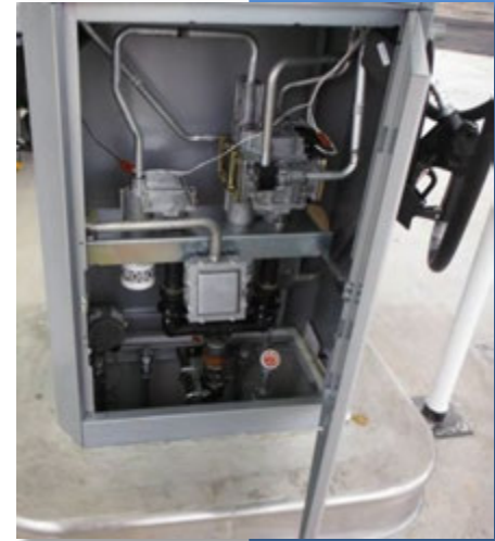
Figure 12.6: Pressurized system dispenser
