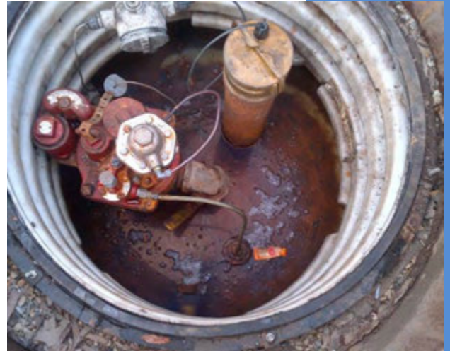
Figure 10.10: Tank top sump with product
