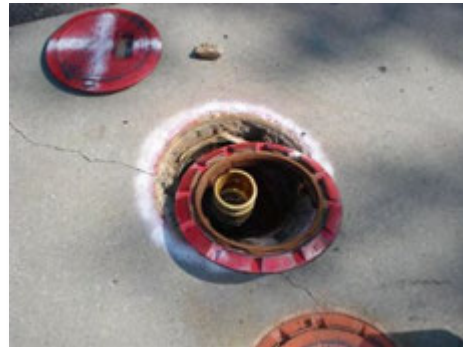
Figure 13.6: Damaged spill bucket
