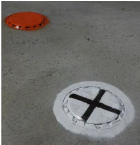
Figure 13.8: Properly colored fill port for unleaded low-grade gasoline (white with black cross) and vapor recovery port (orange circle).
