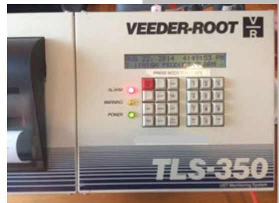
Figure 9.1: Monitoring console in alarm
