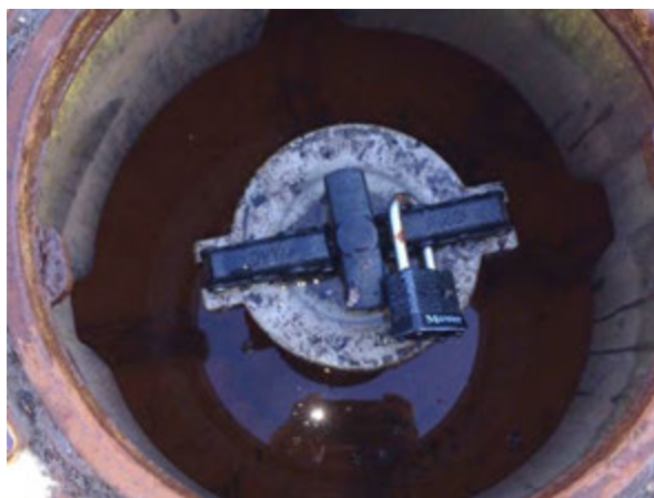
Figure 13.3 Dirty spill bucket in need of cleaning
