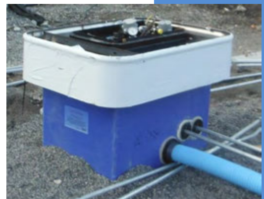
Figure 12.9: UDC with a steel island before burial, showing underground piping and conduit connections.
