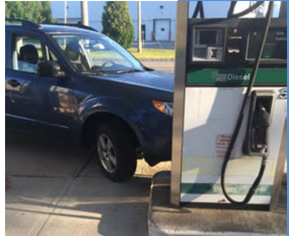
Figure 12.18 Be sure to check your shear valve after an accident such as a vehicle hitting a pump
