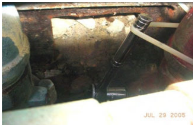
Figure 12.12: Shear valve held open with a socket wrench and zip tie. This, like the shear valve in the previous figure, is a major fire and environmental hazard, and would fail a DEC inspection.
